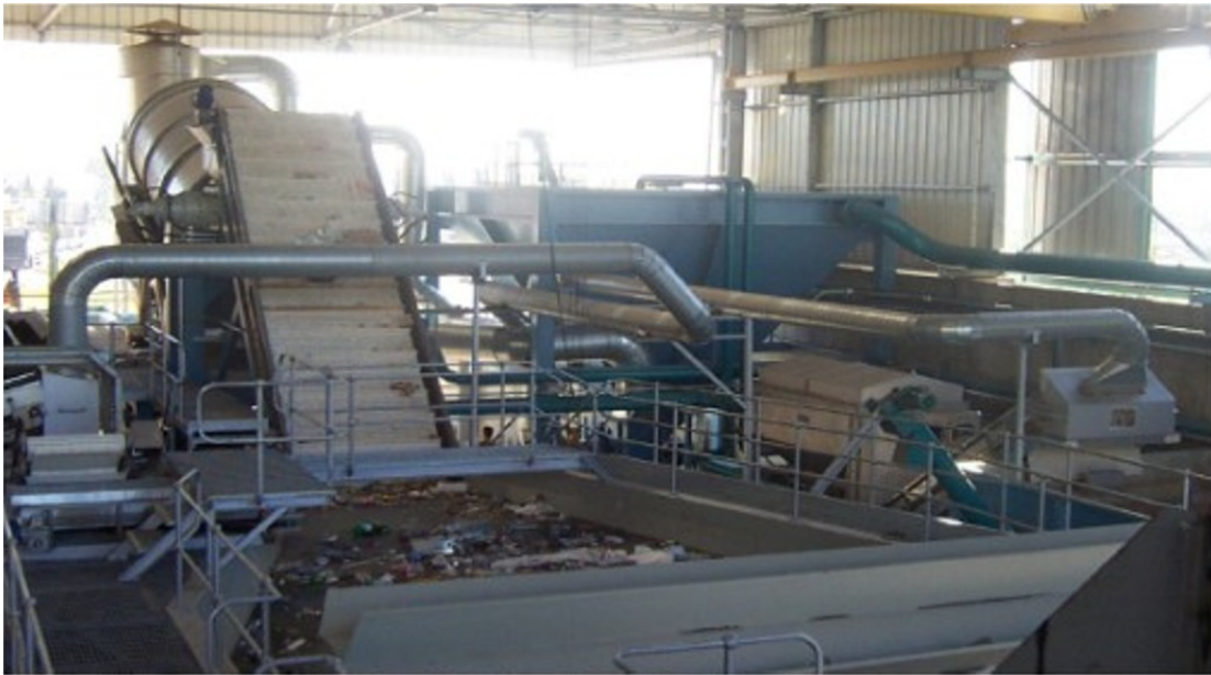
Hydro-Mechanical Sorting systems
